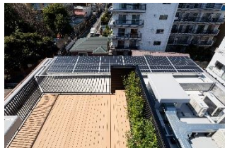
Solar Panels on the Rooftop
